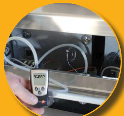
VERIFICA PRESSIONE GAS GAS PRESSURE CHECK
